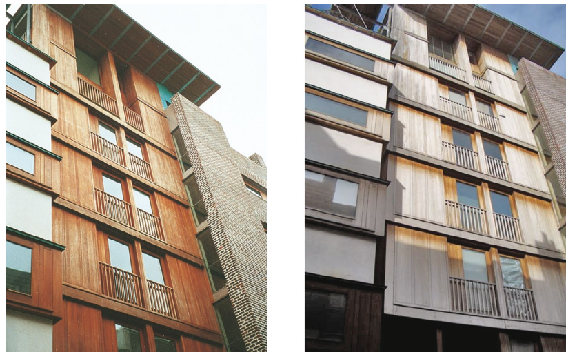
Figure 6: Iroko cladding before (left) and after (right) weathering, Temple Bar, Dublin
